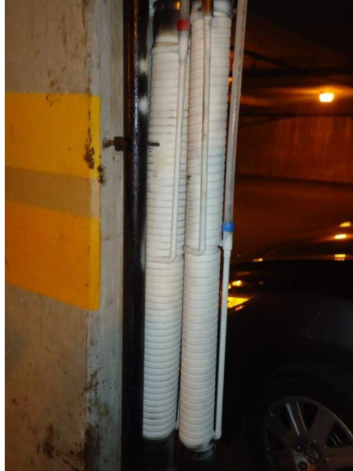
Figure 8 Heat Exchanger at Haro Park
